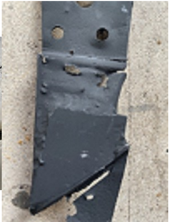
Above: One of the door jambs has extra steel welded into it to compensate for the lack of timber
