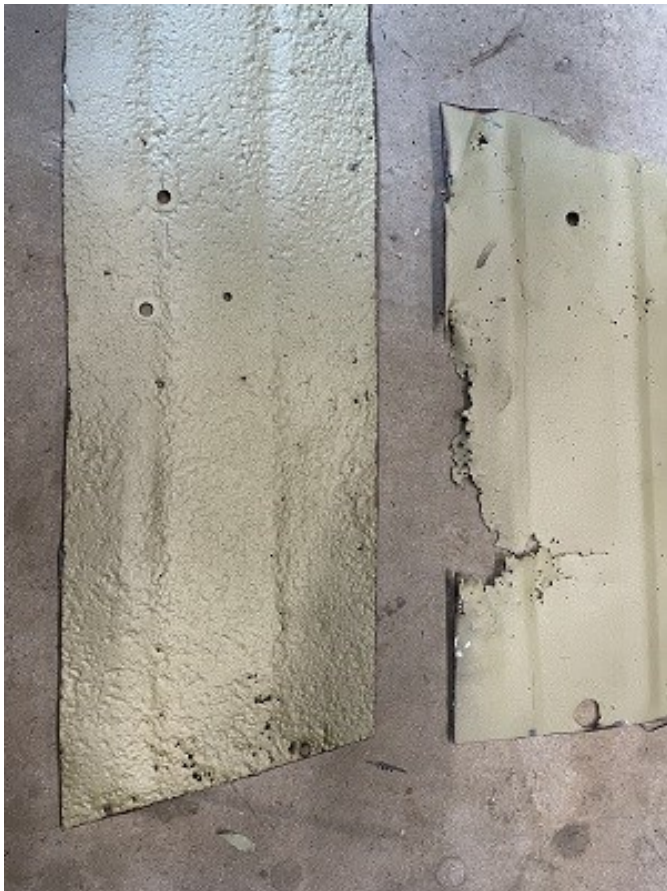
Above: The battery box floor is on the right
